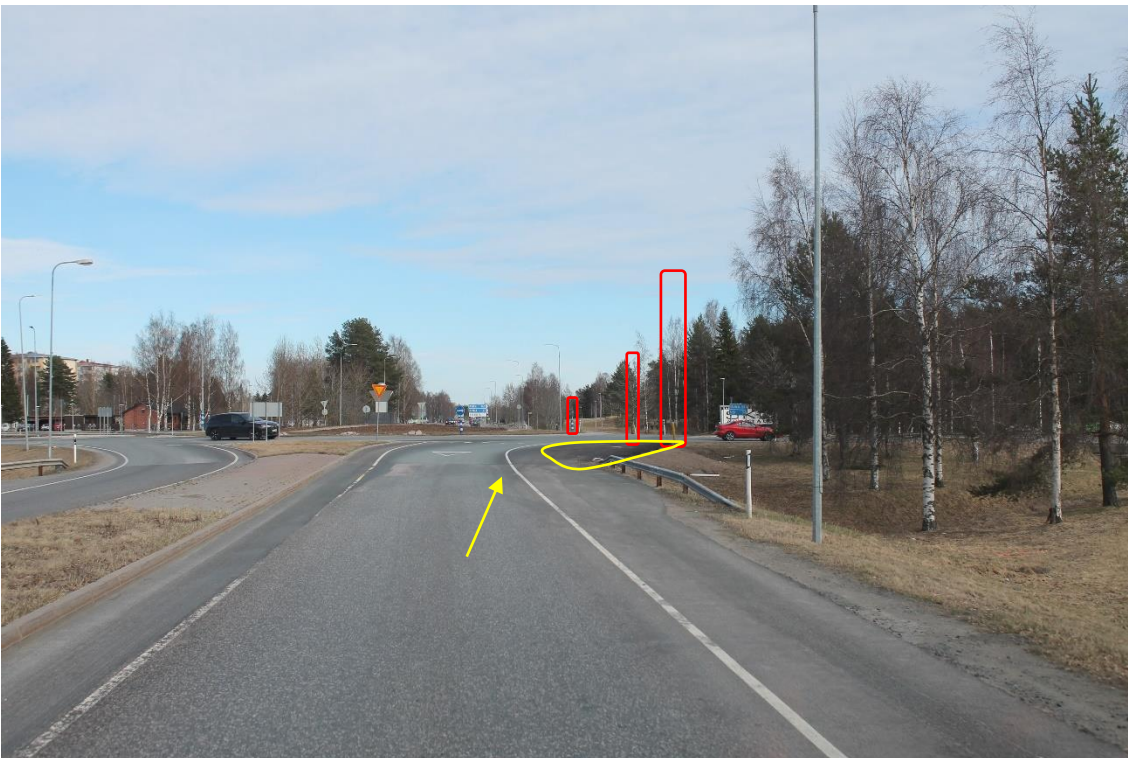
Pos 7/Pic 12. First roundabout on Road 27. https://goo.gl/maps/DPdr3QMEoa45F6Nw8 Continue straight on road 27. Marked signs (one missing) and lamp post (missing) need to be removed. Marked area need to be filled and drivable.
