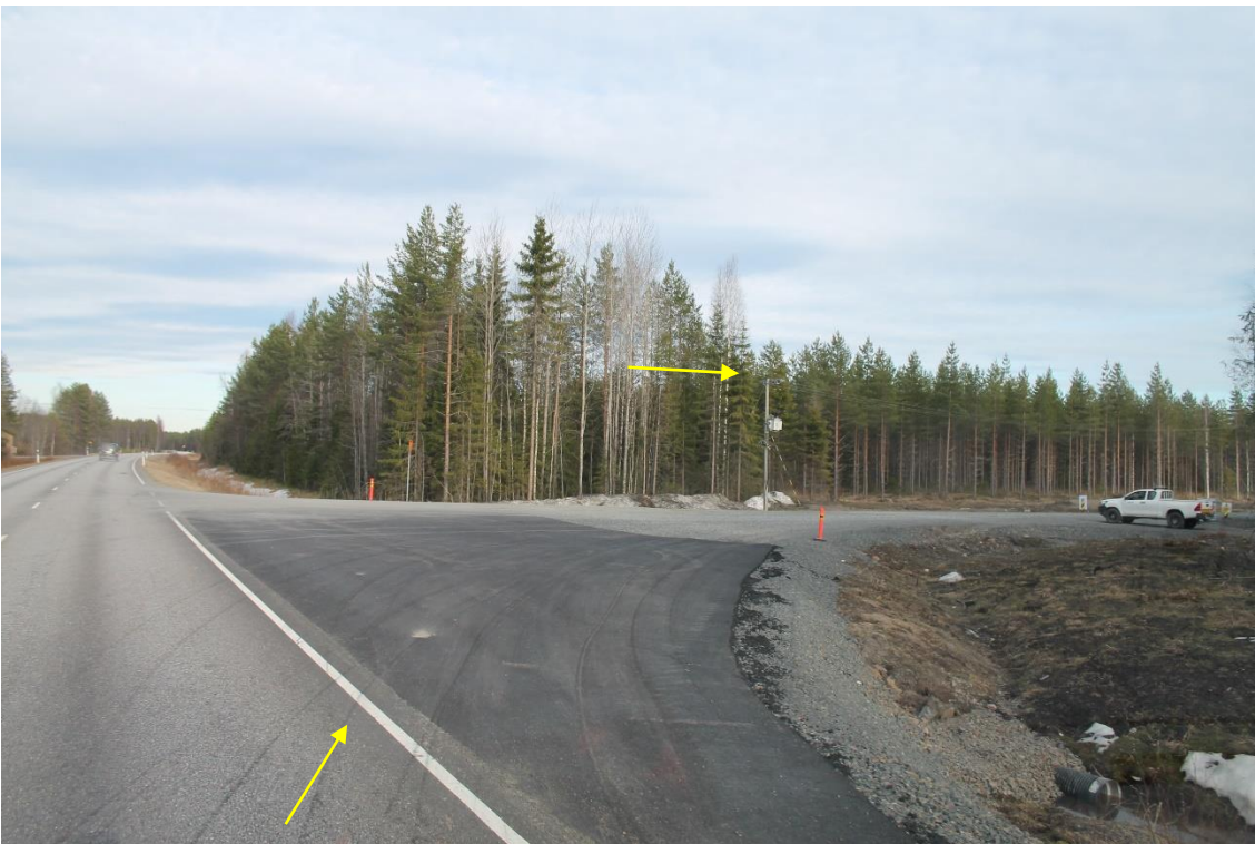
Pos 23/Pic 36. Site entrance. Turning from Road 27 toward Murtomäki site area. Site entrance to be constructed according to turbines suppliers specifications.
