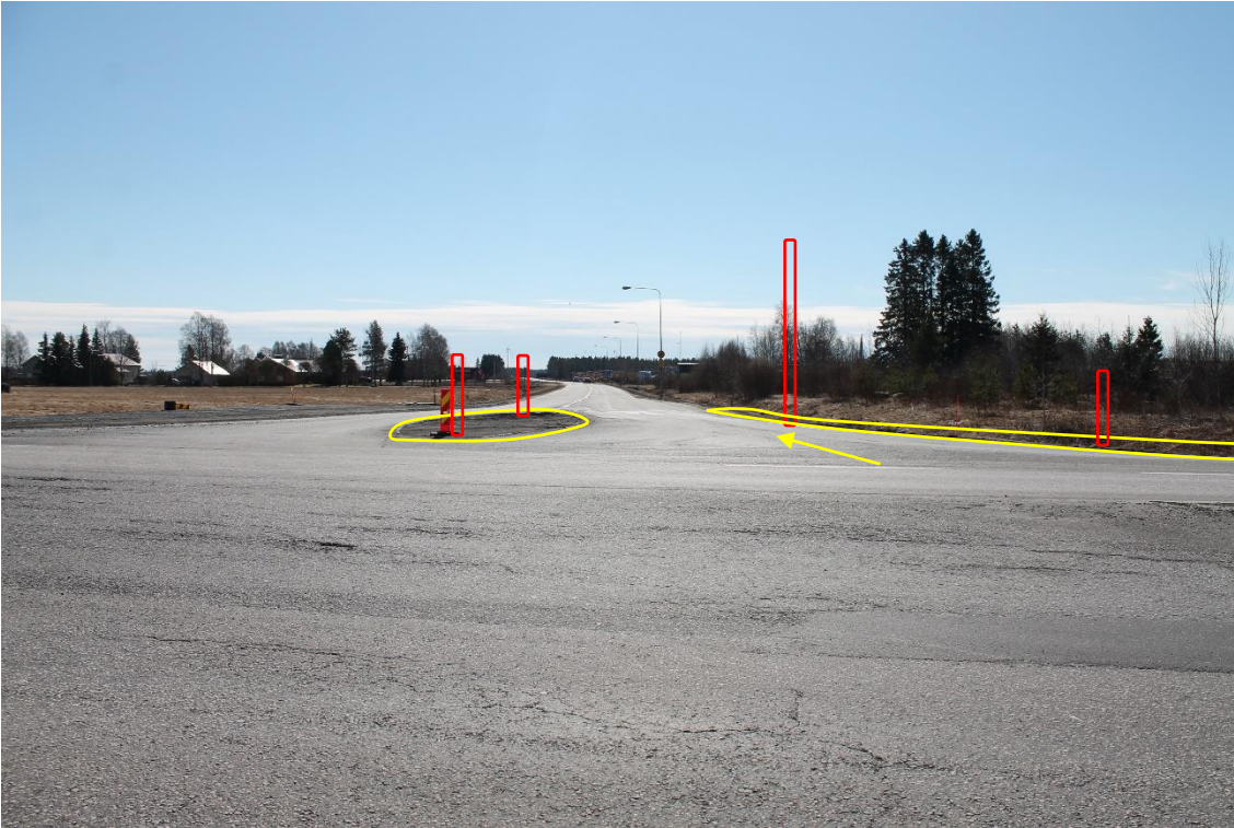
Pos 4/Pic 9. Turning from road 8 toward road 27. Marked lamp post (missing) and signs (missing) need to be removed. Marked areas need to be filled.
