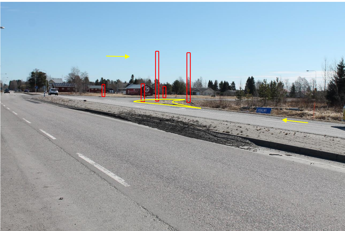
Pos 4/Pic 8. Turning from road 8 toward road 27. Marked lamp posts (missing 2pcs) and signs (missing) need to be removed. Marked area need to be filled.
