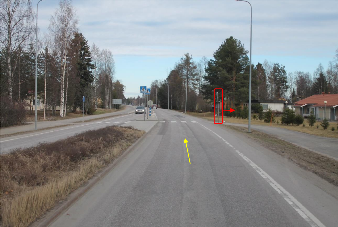
Pos 20/Pic 31. Road 27 in Haapajärvi. Marked sign need to be removed.
