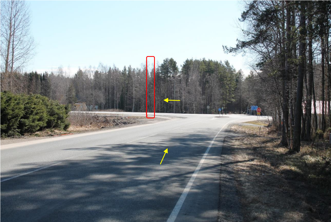
Pos 2/Pic 3. Turning from road 7771 toward road 8. https://goo.gl/maps/ZAwFRpyGBs4upWun6 Marked lamp post (missing) need to be removed.
