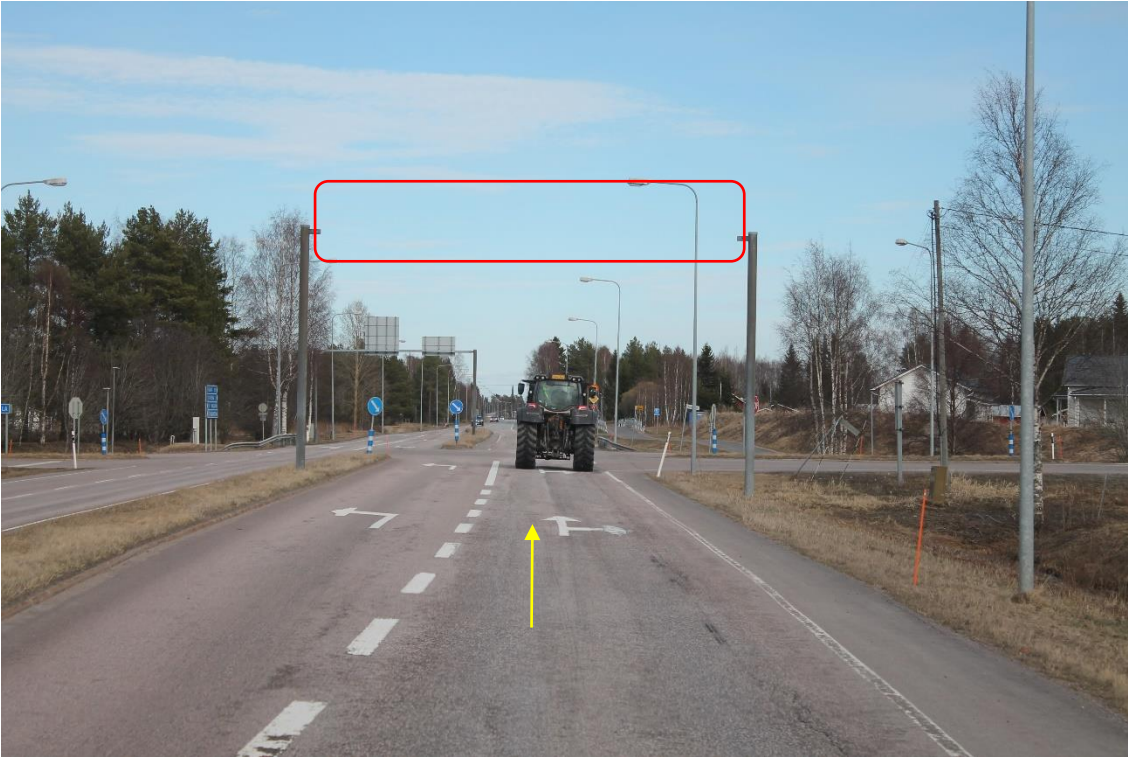
Pos 6/Pic 11. Road 27 in Ylivieska. https://goo.gl/maps/MTkoZGUZLhy1fFs4A Marked portal (missing) need to be removed.
